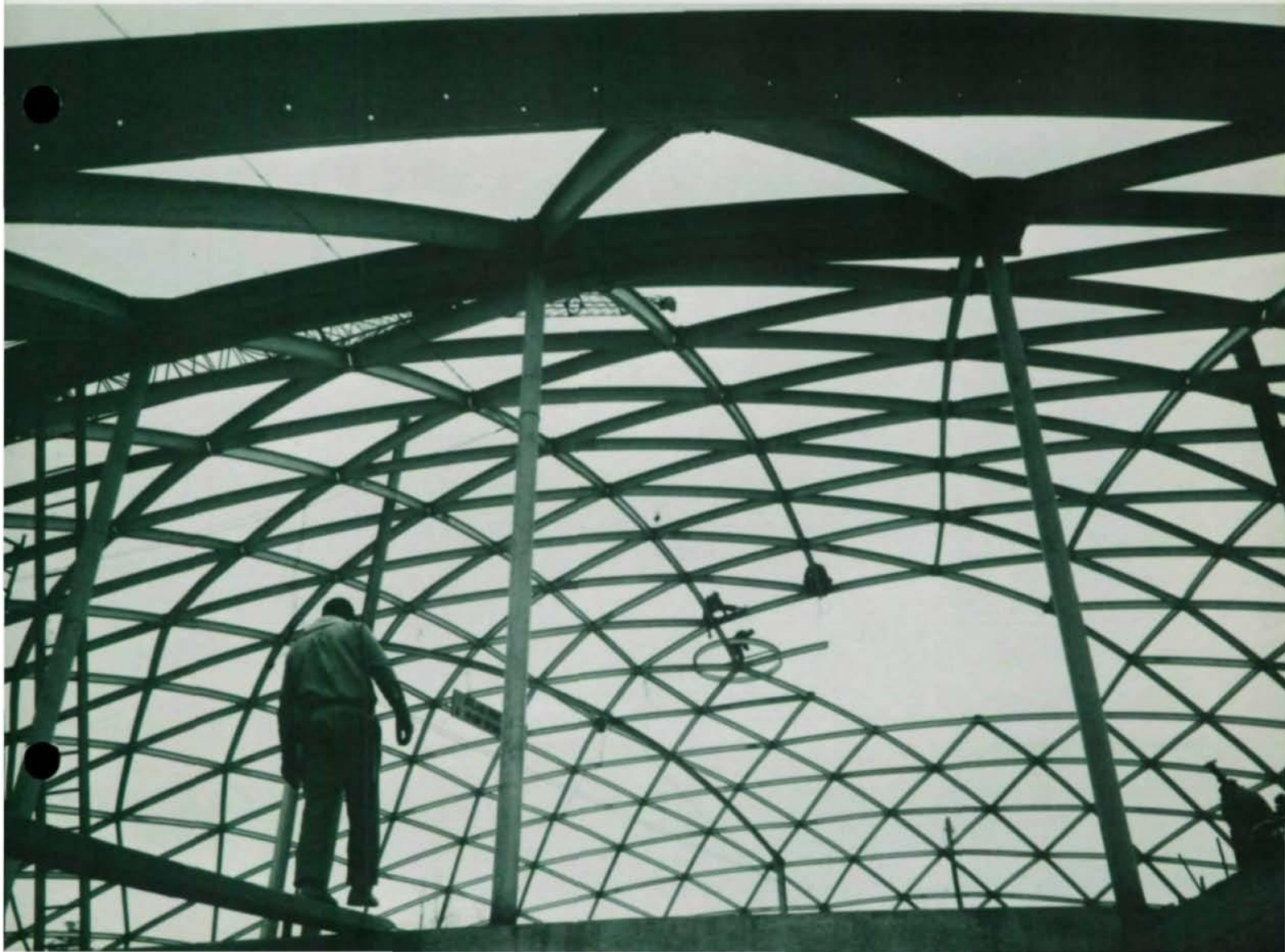
A Study in Patterns as the 8B10 Geodesic Grid Members Near Final Erection.
